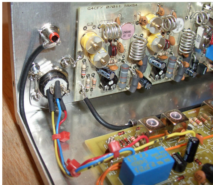
Internal View showing the new wiring Tie wraps keep the new wires tidy
